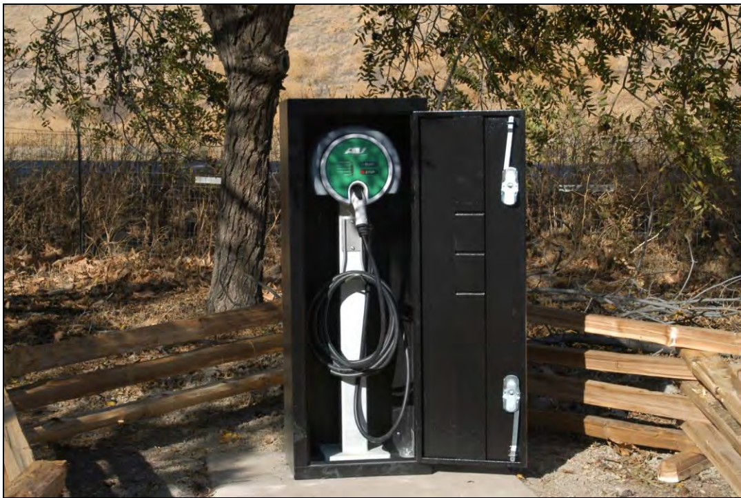
Figure 6. New charging station installed for use by electric dirt bikes.
