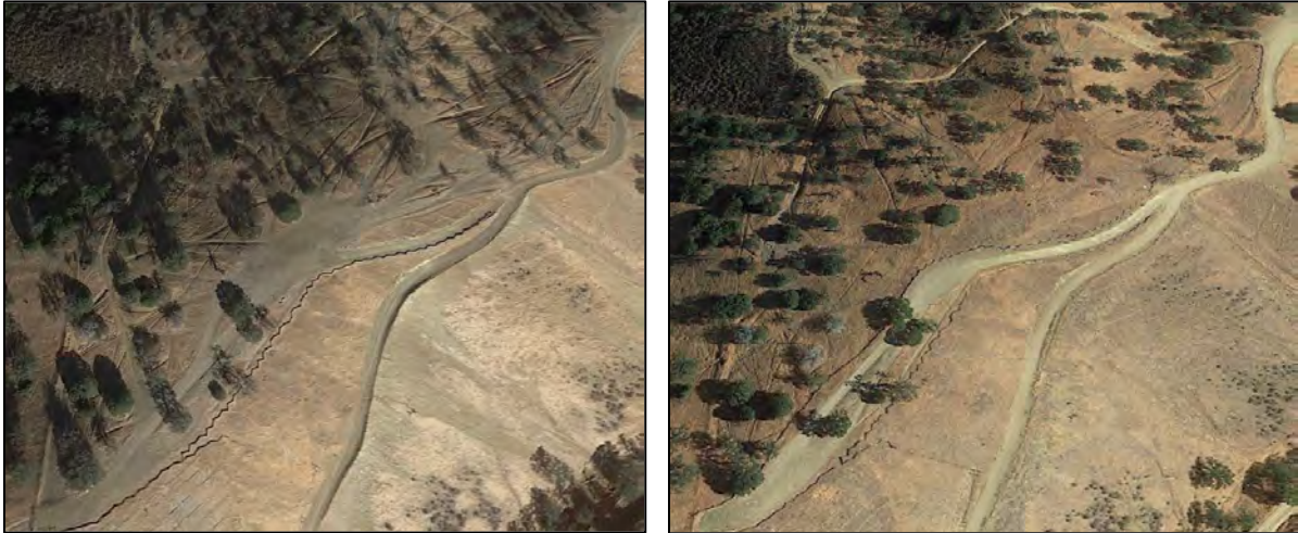
Figure 19: Phase 3 Sub-RMA. The aerial on the left shows the area prior to rehabilitation (Oct. 2015) and the photo on the right is from June 2018 after work was completed.
