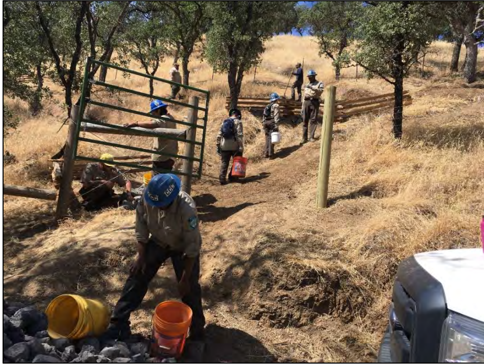
Figure 15 Staff and the CCCs hand-placing rock to prevent erosion on the side of a new trail in Black Bear Sub-RMA. (2018)
