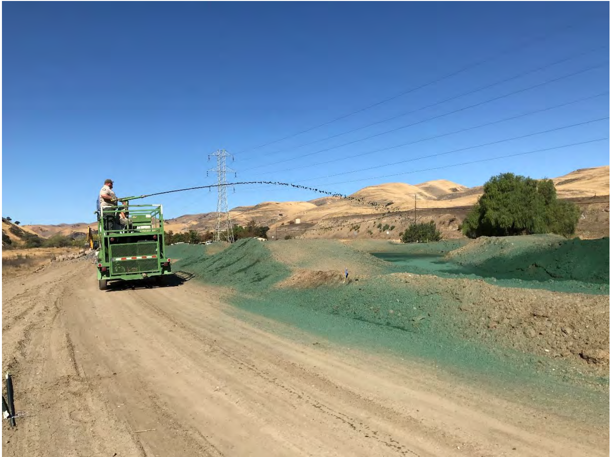
Figure 5 Revegetation Efforts: Hydro-seeding the bare soil of the quad track in preparation of the wet season
